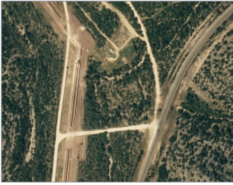
Pipeline construction project with cleared land and pipe laying underway in Val Verde County, Texas
